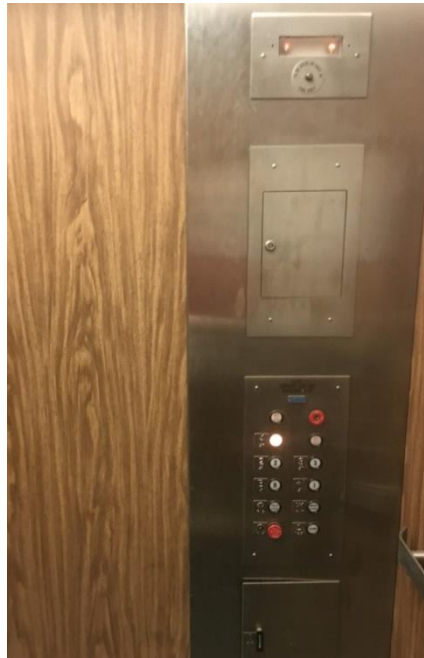
Elevator Control Panel
