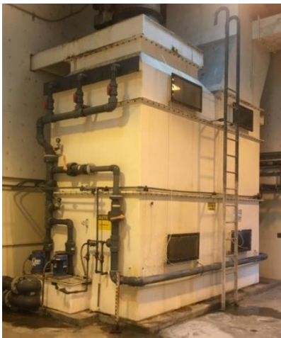
Headworks odor control scrubber
