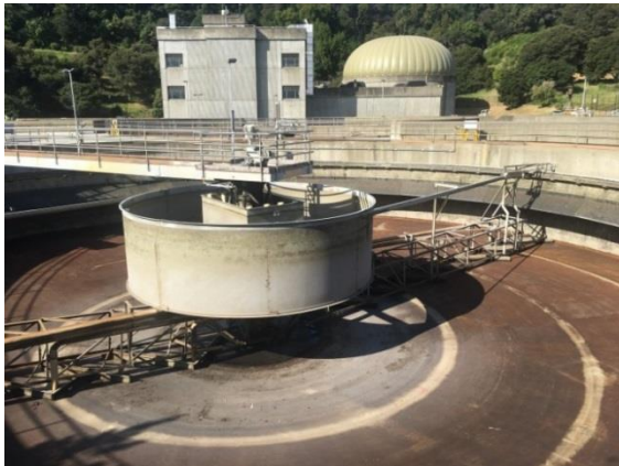
Secondary clarifier internal equipment
