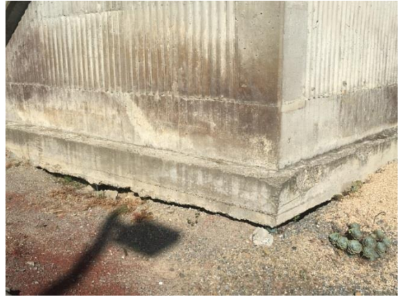
Exposed bottom of process tank
