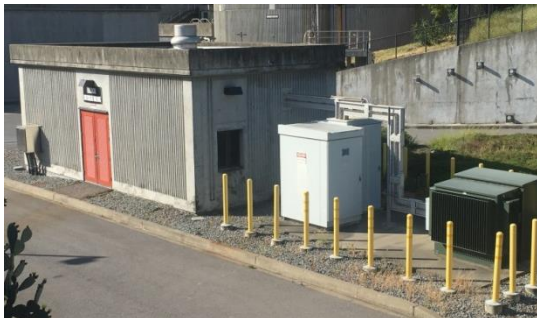
Switchgear building and transformer
