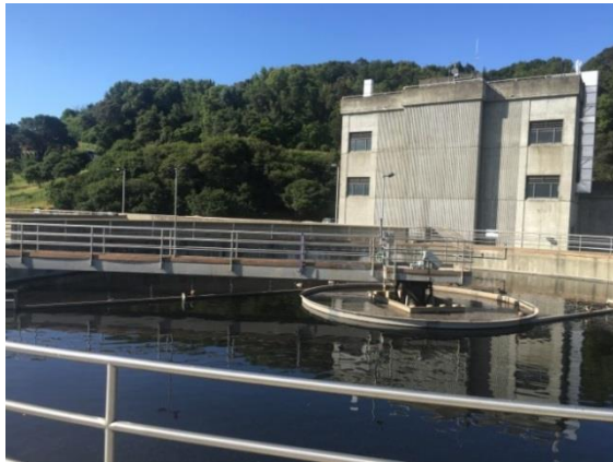
Secondary clarifier in operation
