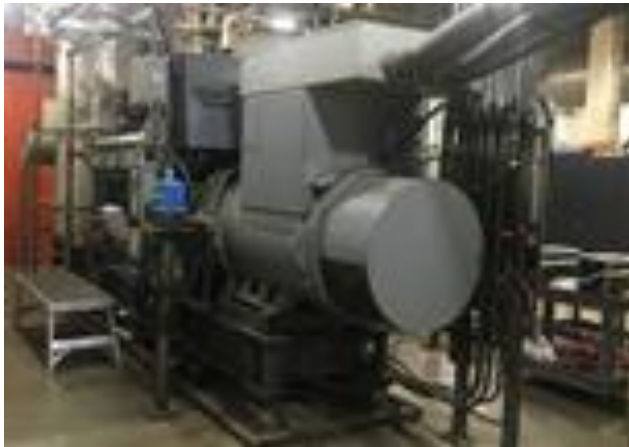
Existing cogeneration system
