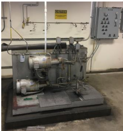
Hydraulic control system
