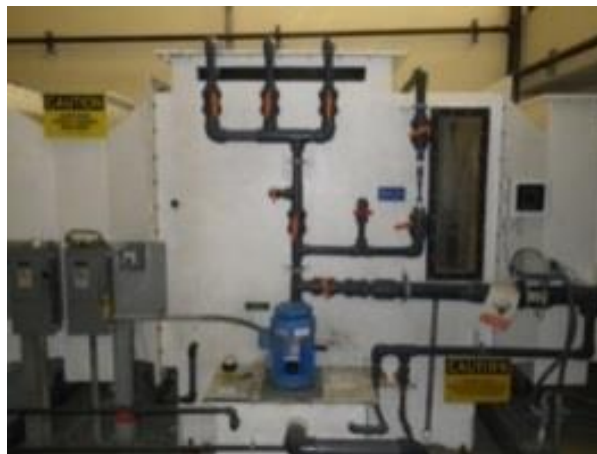
Solids Handling Building odor control scrubber
