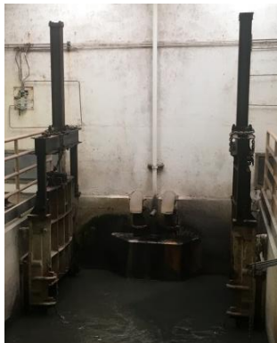
San Rafael and Ross Valley influent gates
