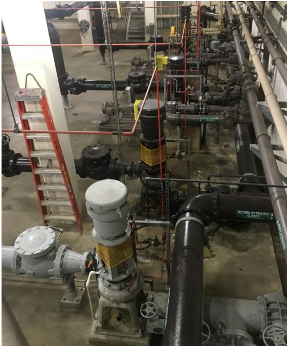
RAS and WAS pumps
